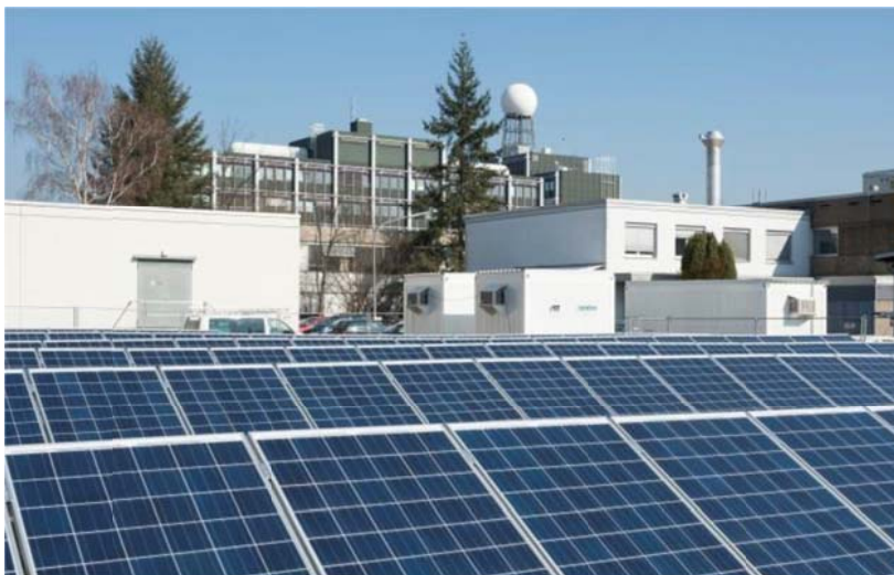
Power from solar parks can be stored in batteries. Balancing of production and demand is one element of the energy turnaround. (Photo: KIT)
